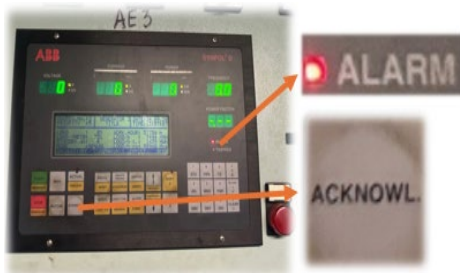
Figure 1 - Generator Control Panel
